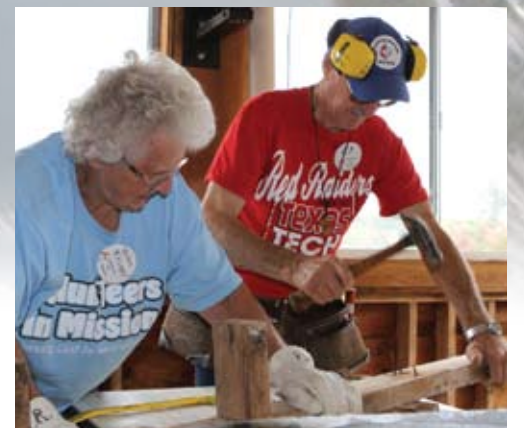
Helen Rhiner and J.P. Holtz of the Wisconsin United Methodist Volunteers in Mission (UMVIM) strip wood from the old Lake Junaluska apartments during their recent mission trip. The materials were donated to Waynesville's Habitat for Humanity.
