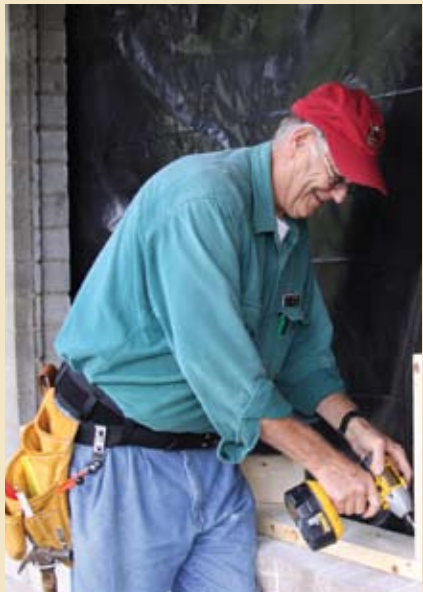
NOMAD volunteer Gary Melvin helps construct window boxes that hold the air/heating units in the newly renovated Sunnyside and Mountain View lodges.
